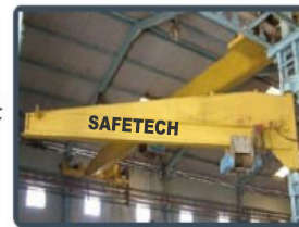
Jib Cranes | Cage Hoists Arrangement
